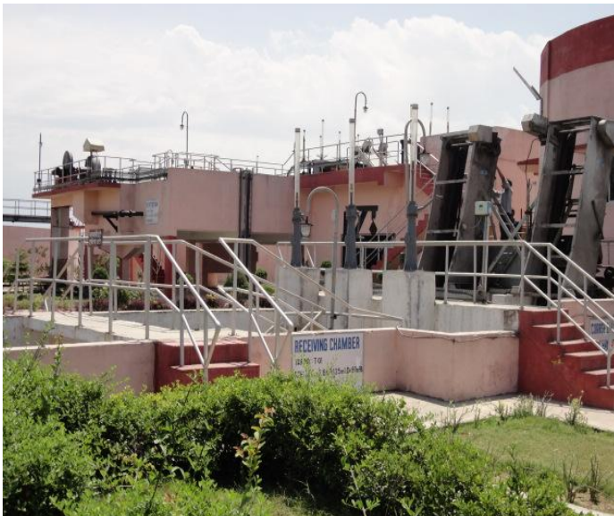
Picture 14: STP at Swarg Ashram
