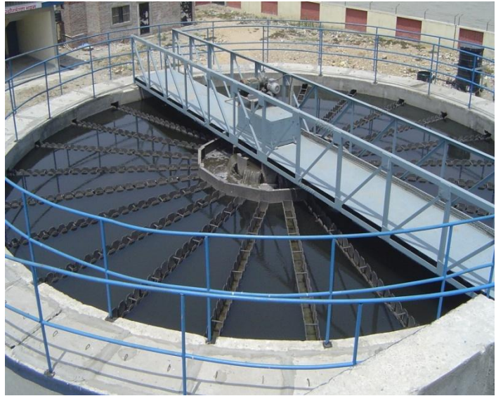
Picture 13: STPs at Srinagar, Uttrakhand
