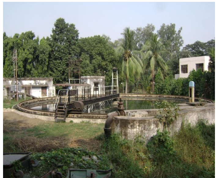
Picture 19: STP at Beur
