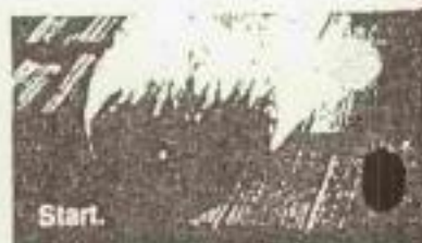
Wood Shakes Fail
