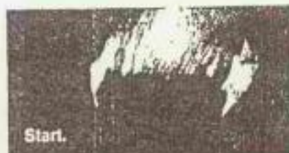
Organic-Based Asphalt Shingles Fail
