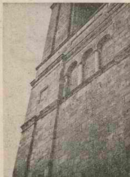
Superficial damage to the facade of the Russian Mission on the Mount of Olives.
