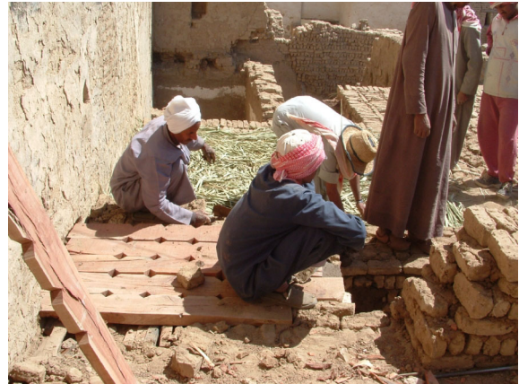
Figure 47 Construction of wooden ventilation grid on the first floor above the entrance to the stairs.
