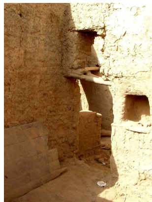
Figure 42 Dilapidated wall between BQur 2 and 5.
