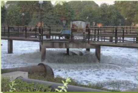
Aeration Chamber of Sewage Treatment Plant (STP)
