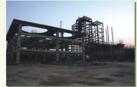
Integrated Waste Management Plant under construction at Okhla by Timarpur Okhla Waste Management Company Ltd.
