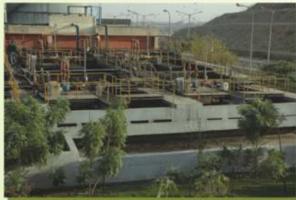
Effluent Treatment Plant (ETP) installed by the Slaughter House, Ghaziipur
